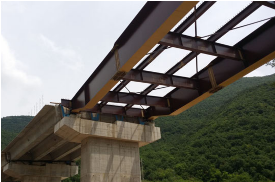
Figure 4.3: Girders installation. Visit to the ongoing works in the road between Perugia and Ancona, Italy.
